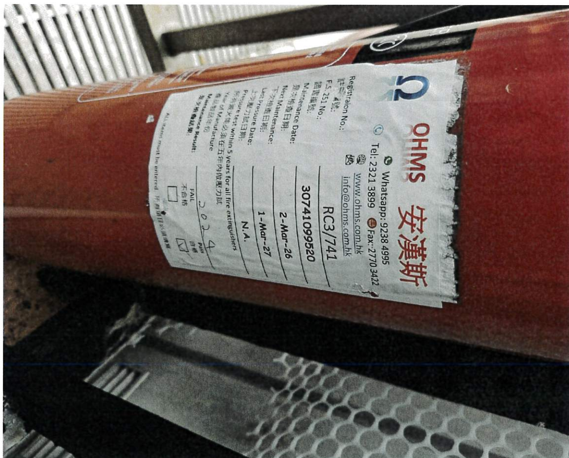
Installed Fire Extinguisher Information
